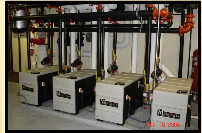
Multiple Boilers – 199,000 BTU each
