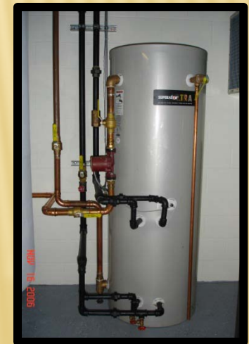
Typical Indirect Water Heater
